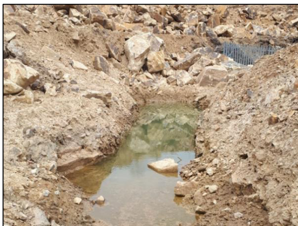
Standing water in the north of the site.
